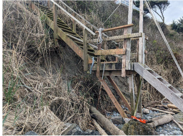
Photograph 4. Erosion observed at toe of steep shoreline slope under existing beach stairs, view to the southwest.
