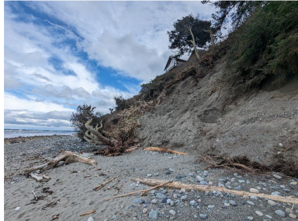
Photograph 9. Landslide on adjacent property, about 50 feet west of Site, view to the east.
