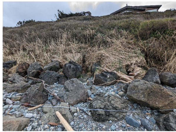
Photograph 2. Bulkhead along the shoreline north of the residences, view to the south.
