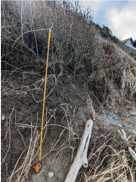
Photograph 6. Erosion behind area of missing face rocks, view to the southwest.
