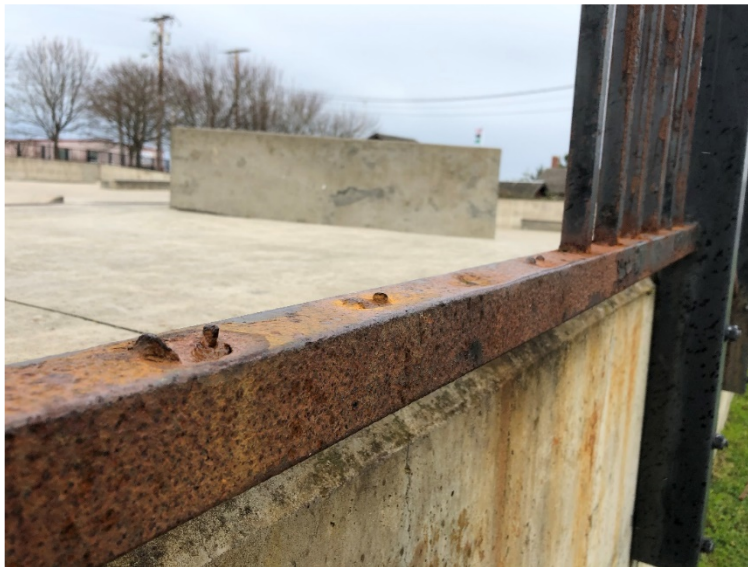
Photo of Typical Corrosion
