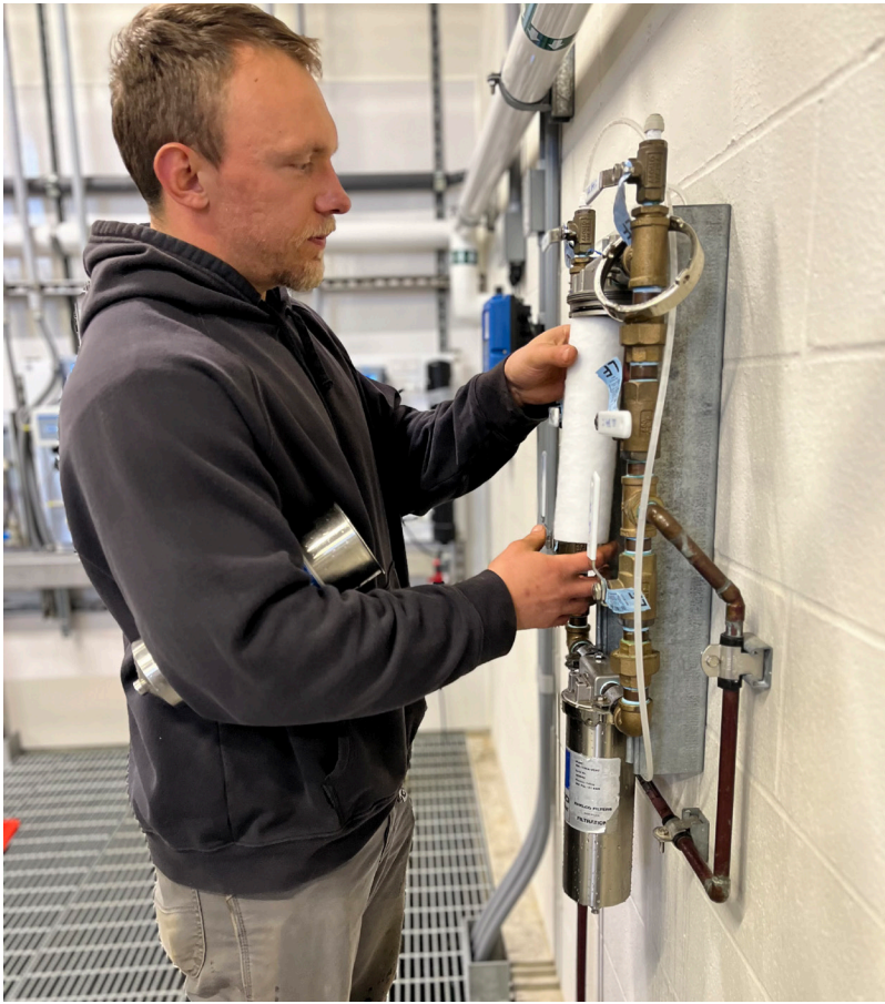
Above: Operator performing preventative maintenance at the Water Treatment Facility. Below: Membrane filtration equipment.
